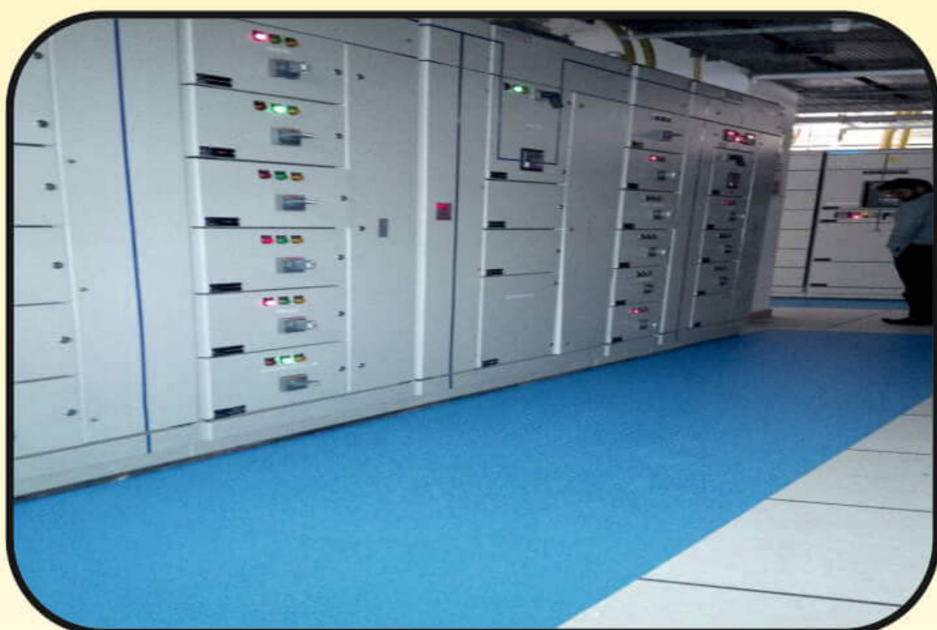
ELECTRICAL INSULATING MATS
